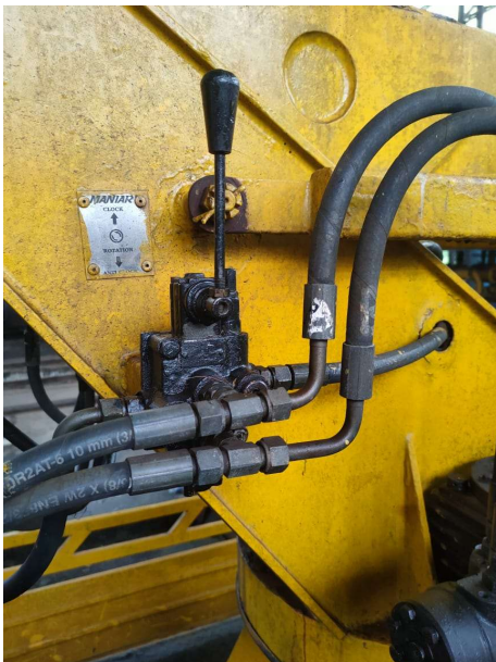
Control valve of the radial
